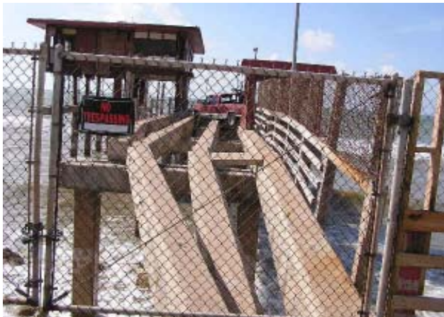
A fishing pier on Seawall Blvd smashed by Ike
